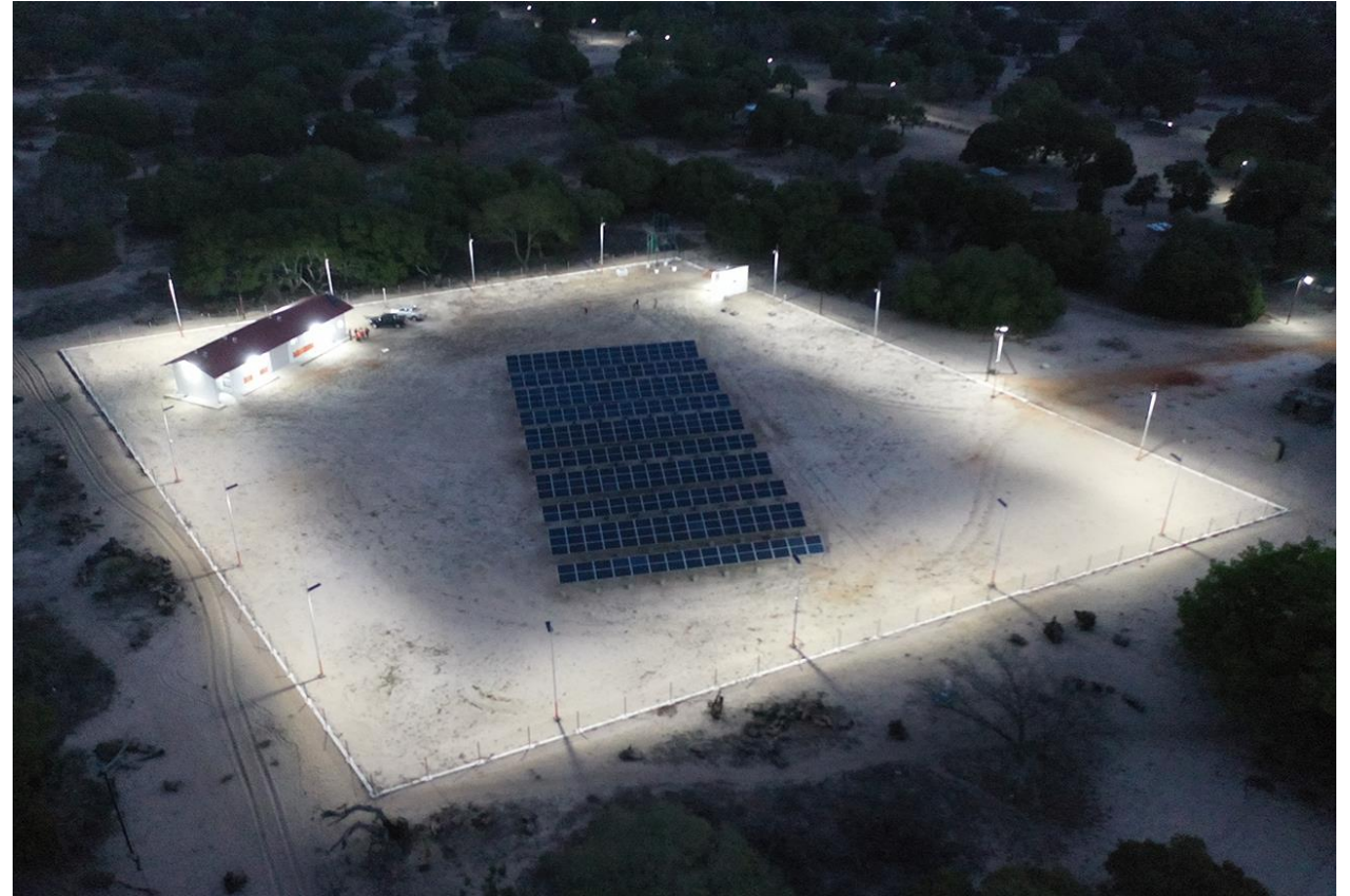
Alto-Changane 200kWp solar PV mini-grid, Alto Changane, Chiobuto, Gaza Source: FUNAE (2021)
